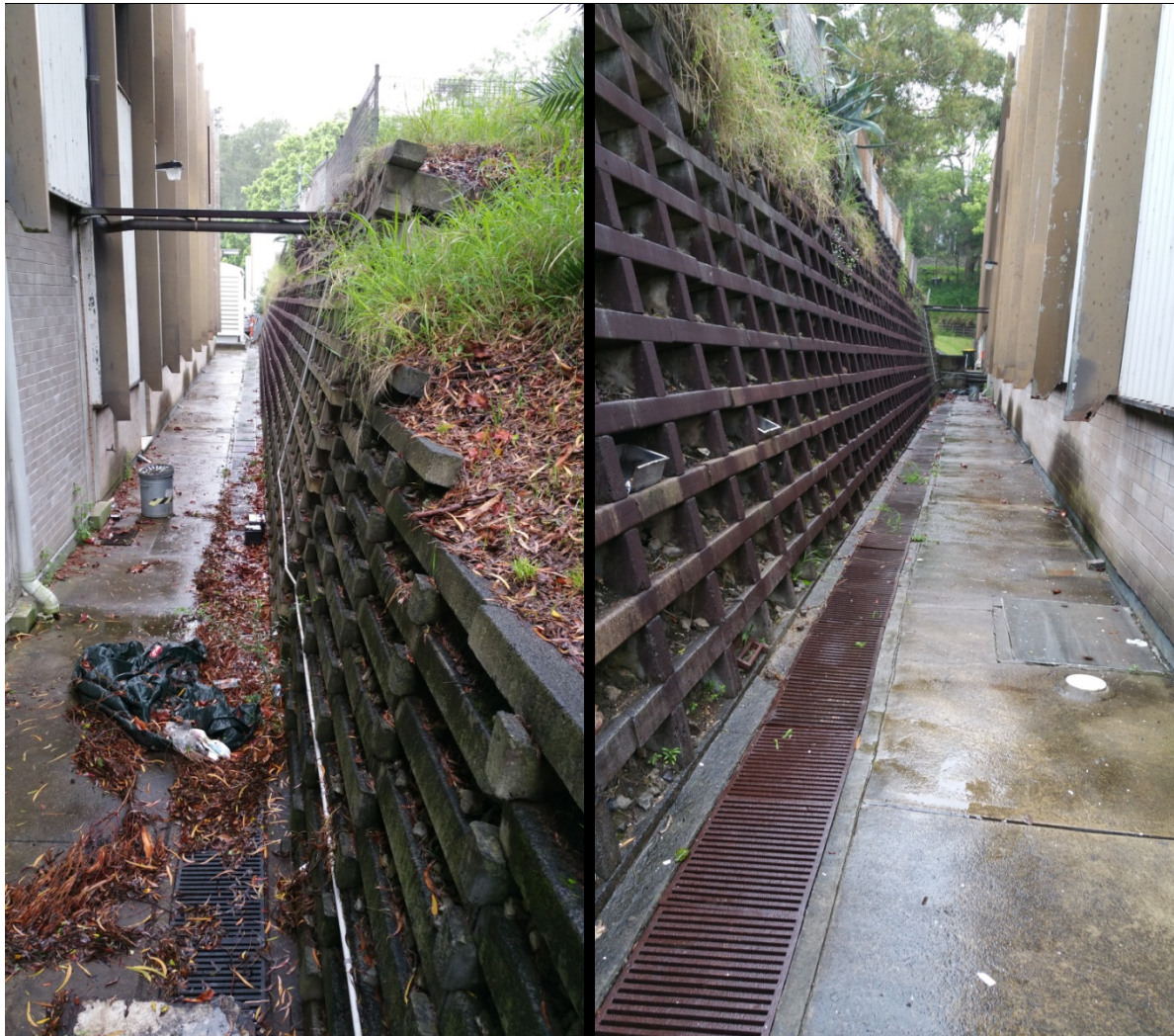
Figure 3: Existing Crib Retaining Wall along Eastern edge of existing NBN building (looking north, looking south)
